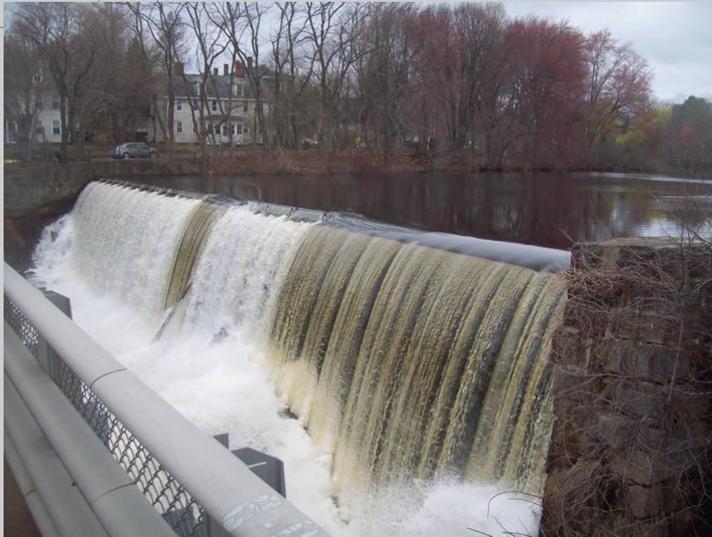
SAXONVILLE LEVEE (ACCREDITED)*
